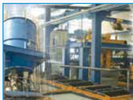
Mini Autoclaved Aerated Concrete (A.A.C. Plant)
